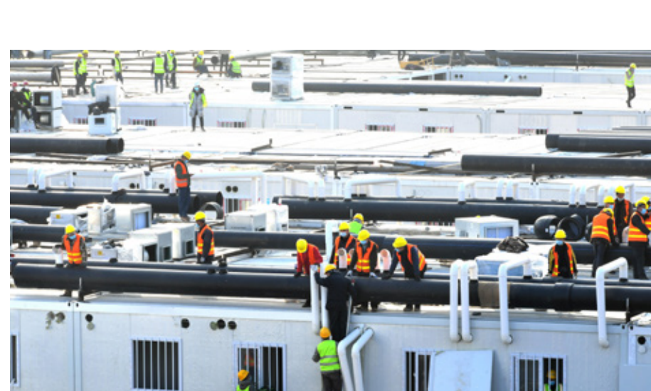
Workers at the construction site of Leishenshan hospital in Wuhan, China, February 2020. Source: An Yuan / China News Service via Getty Images
