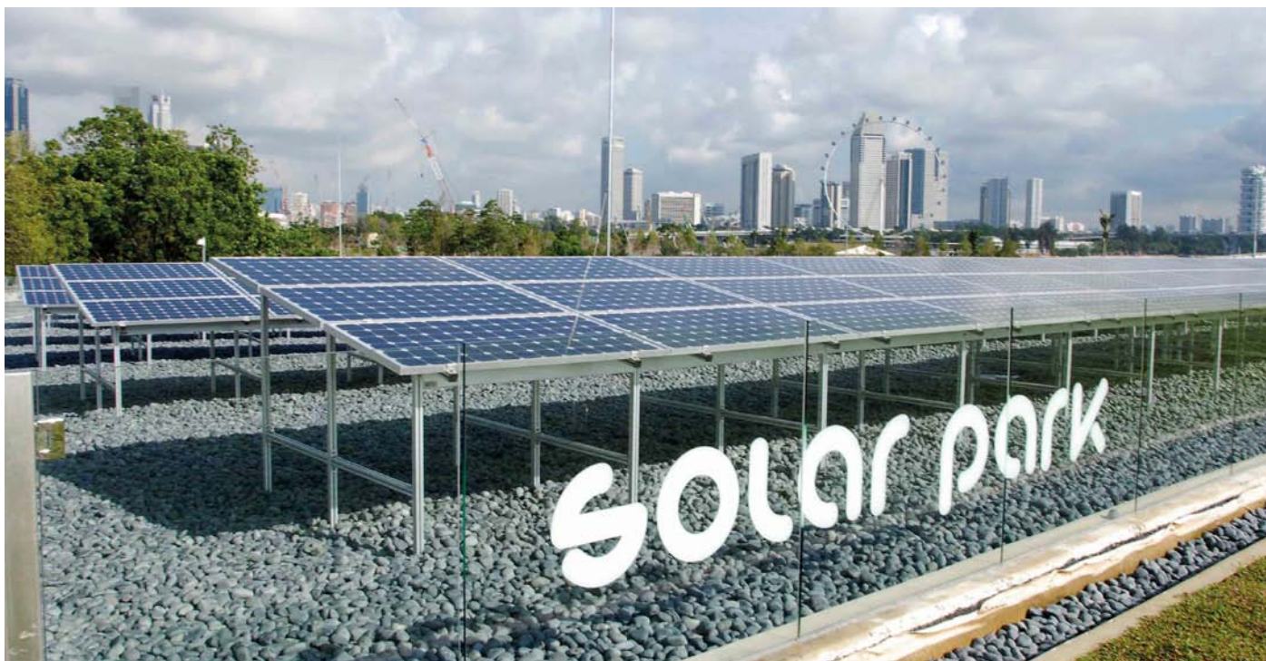
The solar park in Marina Bay is the largest field of solar panels in Singapore, generating 50 per cent of the daytime electricity needs of the Marina Barrage facility. Photo courtesy of PUB, Singapore's national water agency.
