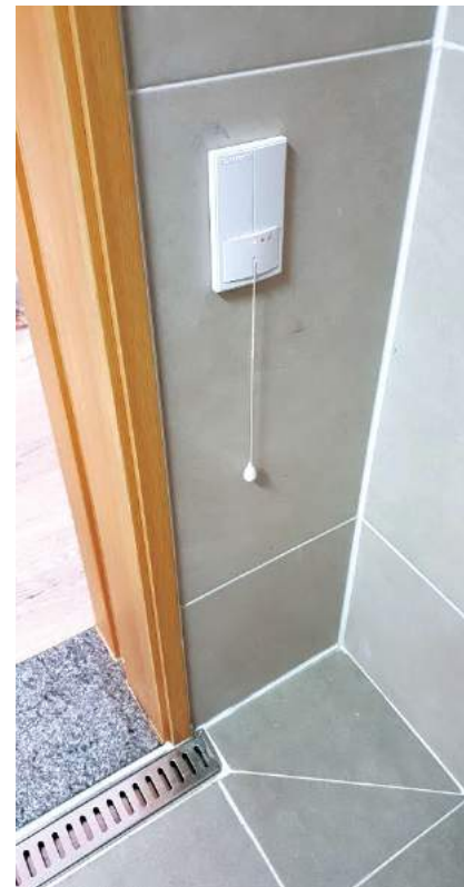
Emergency alarm installed in the bathroom.
