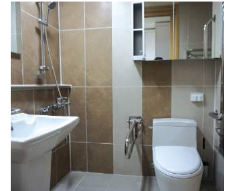
Toilet fitted with grab bars.
