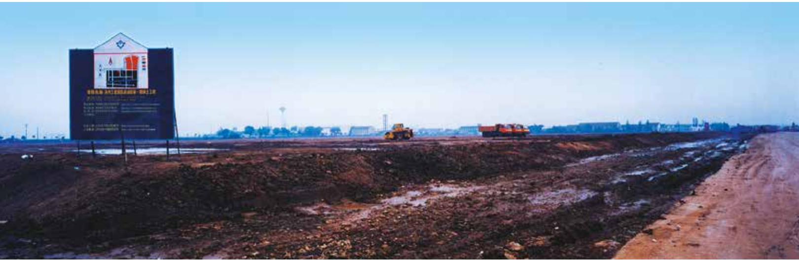
Launch of the SIP's Phase One development on 12 May 1994; landfilling truck fleet in 1994; the SIP's landfilling project
