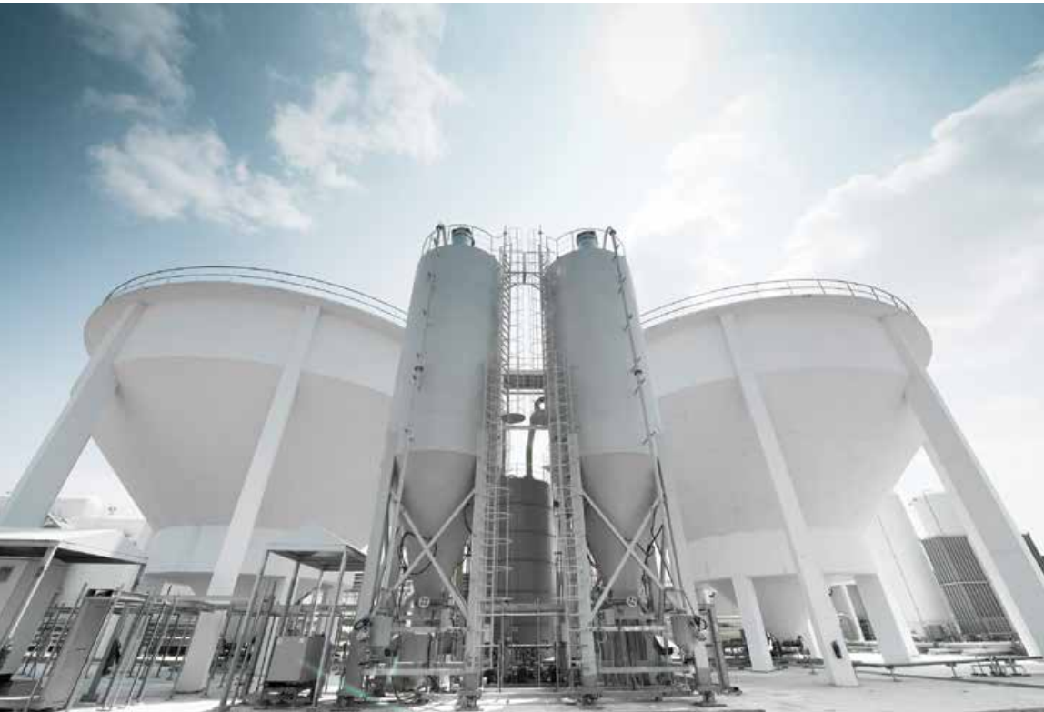
The two desalination plants in Singapore are designed, built, owned and operated by the private sector. Source: Hyflux Ltd
