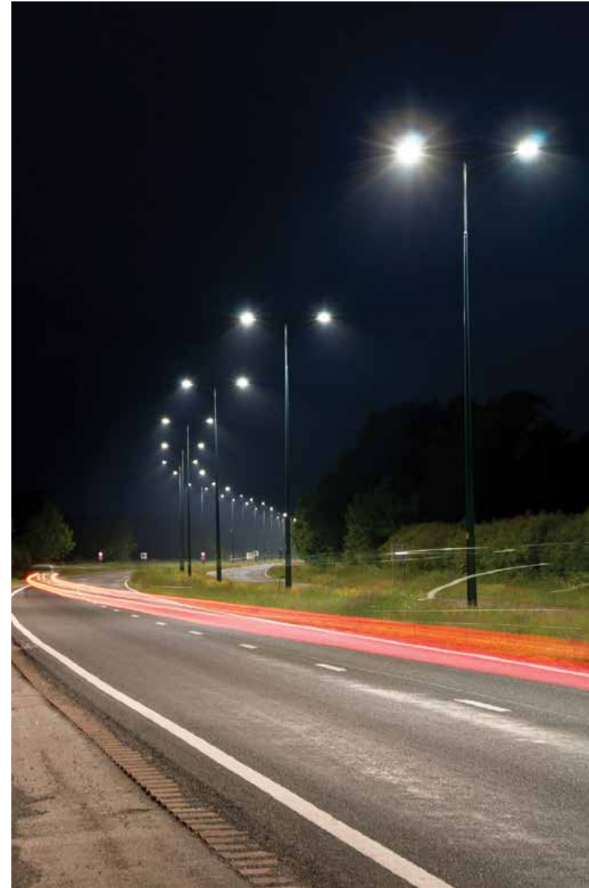
New cost- and energy-saving LED street lamps. Source: ENGIE
