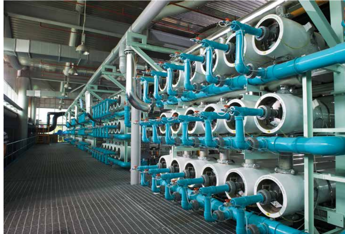
NEWater is produced using advanced membrane technologies to purify treated used water. Source: PUB, Singapore's National Water Agency
