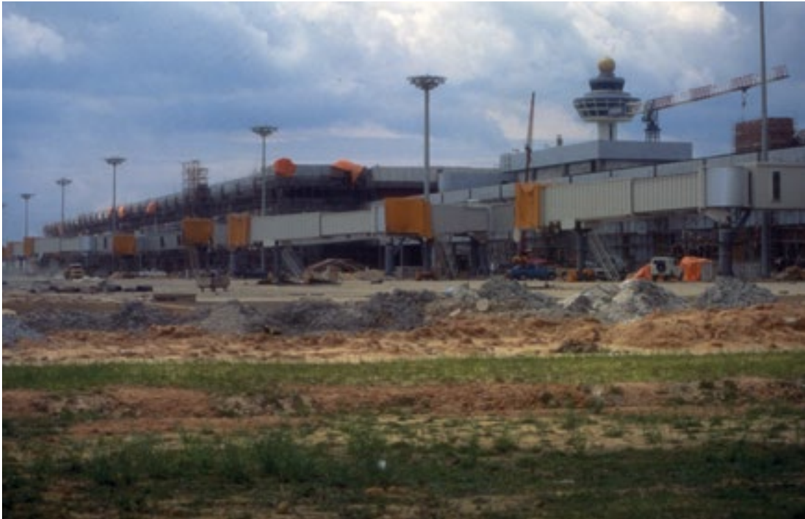
Changi Airport under construction, November 1980. The airport officially opened on 29 December 1981. (Civil Aviation Authority of Singapore Collection, courtesy of National Archives of Singapore)
