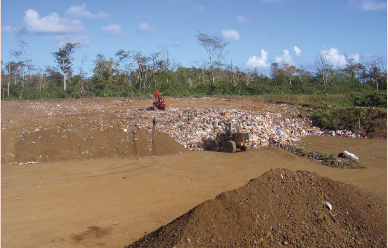
Deployment of the Fukuoka Method to a waste landfill site. Image: Fukuoka City
