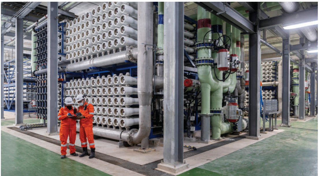
Aerial shot of Marina East Desalination Plant (MEDP) and reverse osmosis system. Image: Keppel Infrastructure
