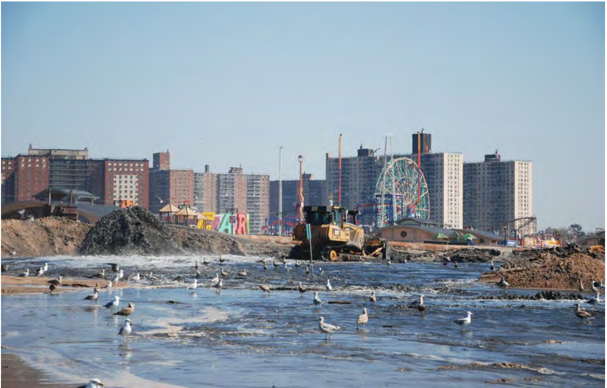
Crews work to restore the beach at Coney Island in New York City and replace sand loss caused by Hurricane Sandy. Image: US Army Corps of Engineers / Flickr
