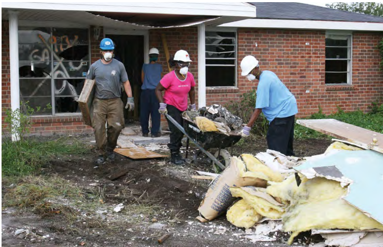
Non-governmental organisations (NGOs) and volunteers played a crucial role in rebuilding homes and communities in New Orleans after Hurricane Katrina. Image: Corporation for National and Community Service Photo
