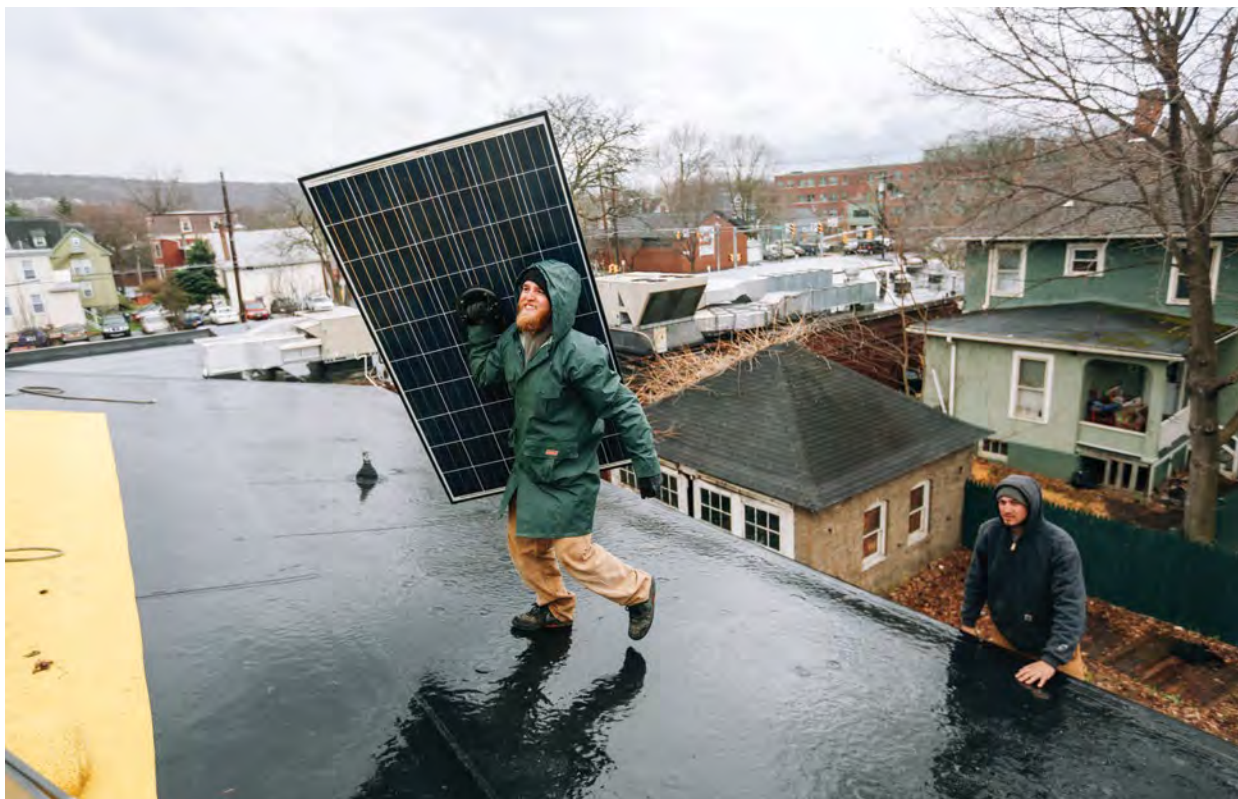
Installation of affordable solar solutions for residents in upstate New York in progress. Image: Stephen Yang / The Solutions Project / Flickr
