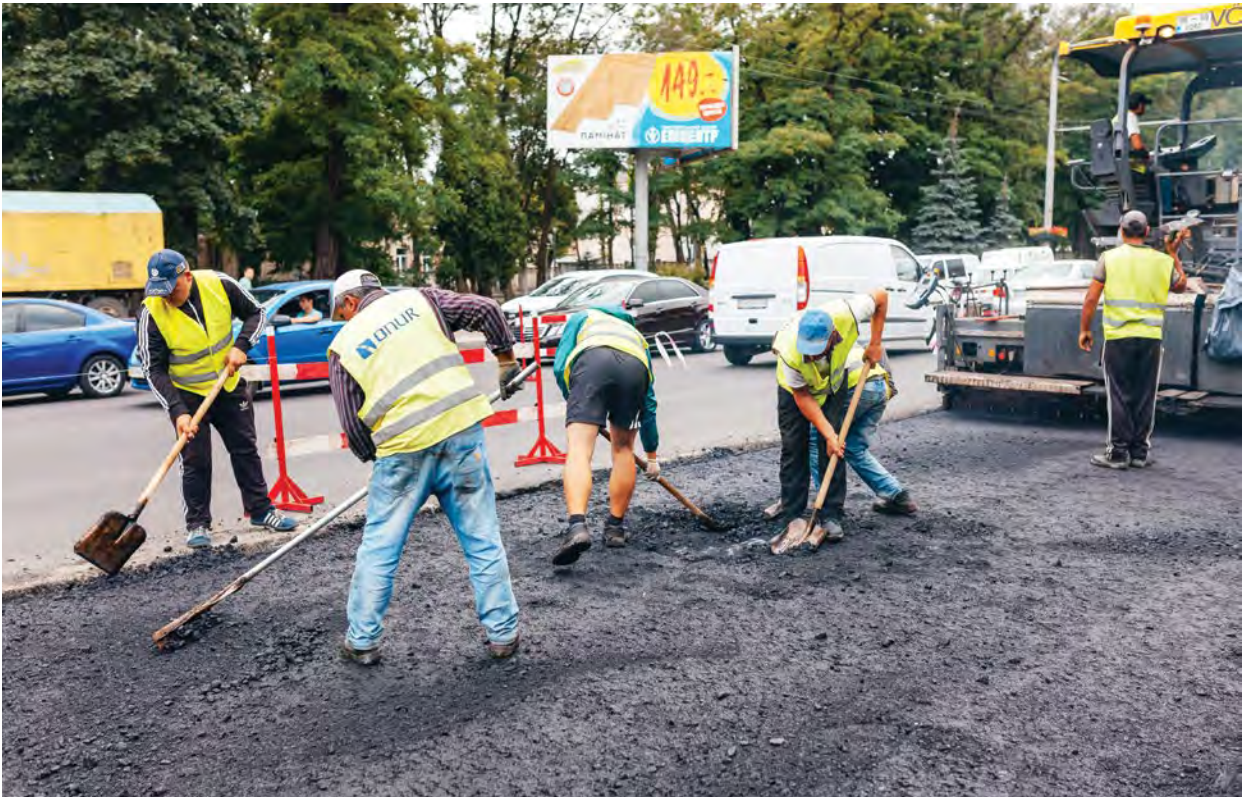
Seoul shares 'Clean Construction System' practices with the Ministry of Infrastructure of Ukraine, which was applied in a road reconstruction site in Kyiv. Image: Andrey Krepkikh / UNDP in Ukraine
