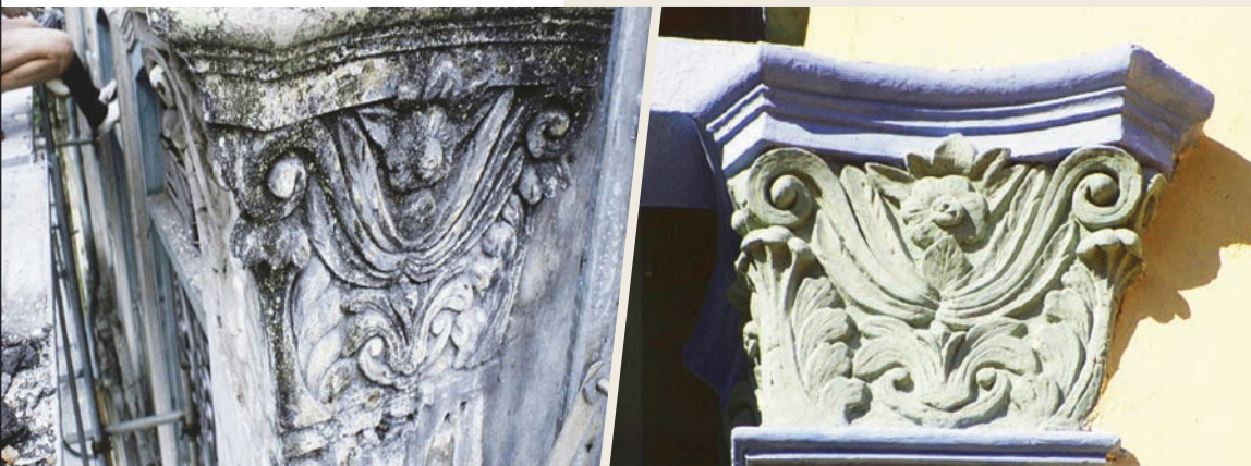
Details of a column at 53 Armenian Street before (left) and after (right) restoration in 1988. Courtesy of Didier Repellin.
