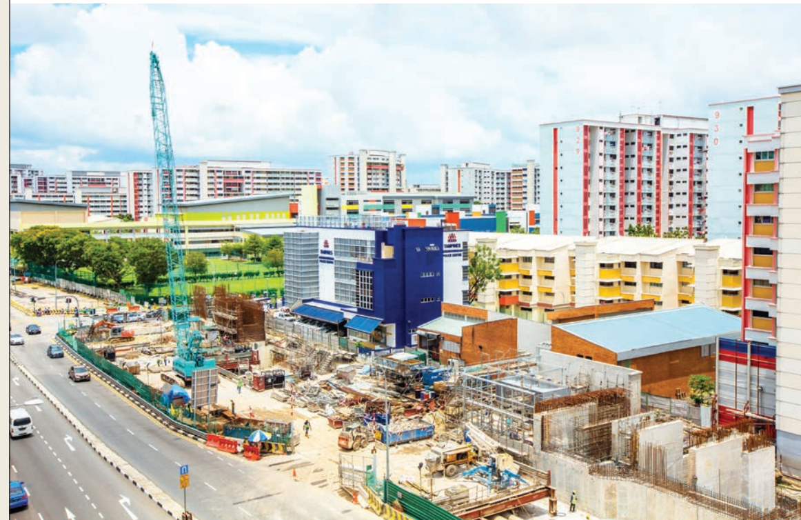
Construction of Tampines West Downtown Line MRT Station close to an HDB estate.
